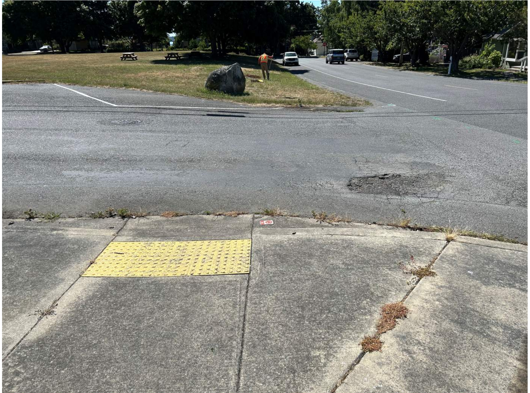
Existing Conditions: Walker Street / Jefferson Street- No Sidewalk along Park, Failed Pavement
