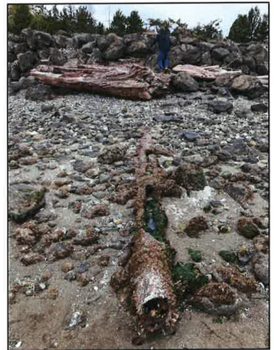
PHOTO SHOWING EXISTING DETERIORATED STORMWATER PIPE AND OUTFALL CONDITION
